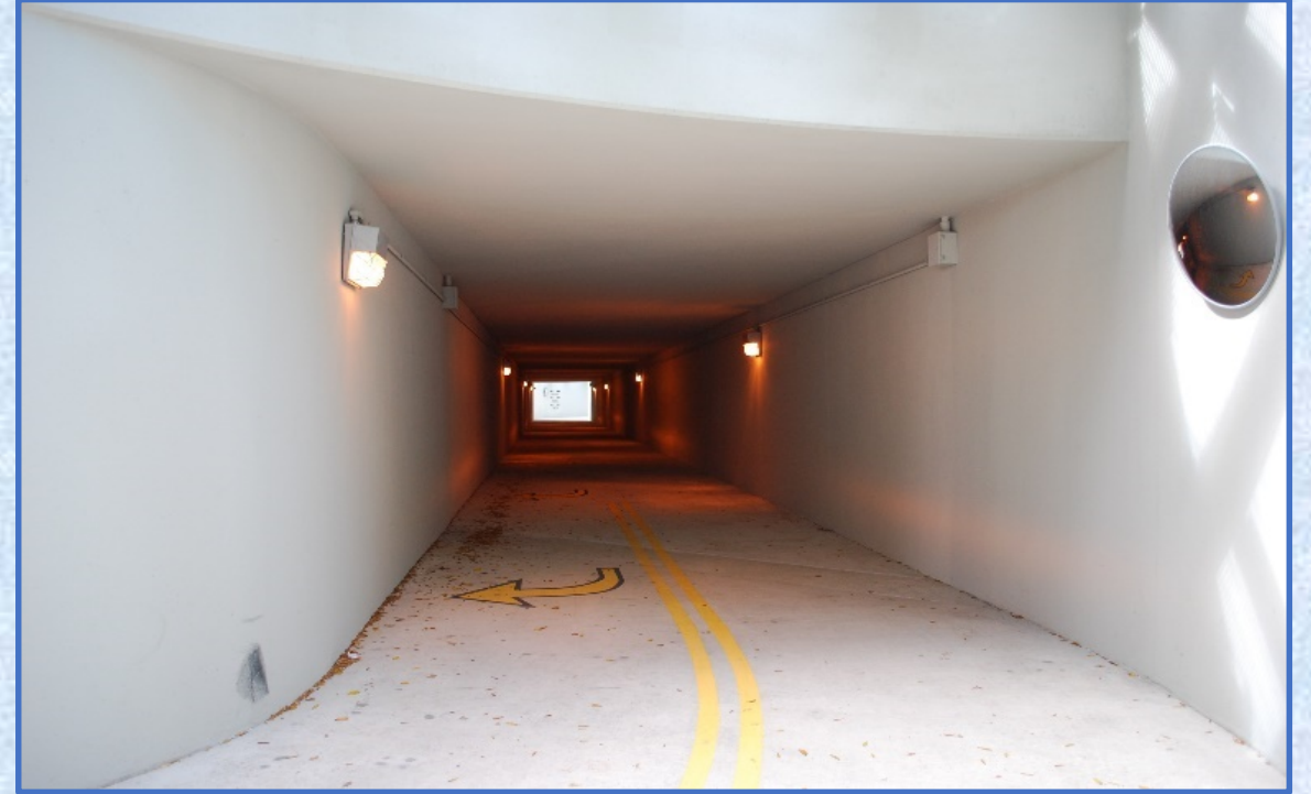
Mirrors, Interior Lighting, Directional Arrows and Delineation Striping
